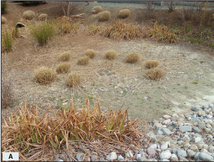
Examples of failing bioretention and swales due to insufficient operation and maintenance.
