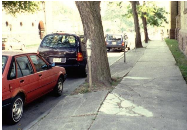
Trees planted in severely limited soil volumes die young unless their roots are able to break past compacted soils into an adequate volume of useable soil. This often results in dangerous sidewalk heaving.
