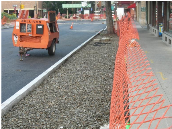
Renovation of this street and sidewalk in Ithaca, NY, provided an opportunity to use CU-Structural Soil® as a 36" base course for a replaced segment of sidewalk. This renovation allows the roots of this existing tree to escape its tree pit confines.
