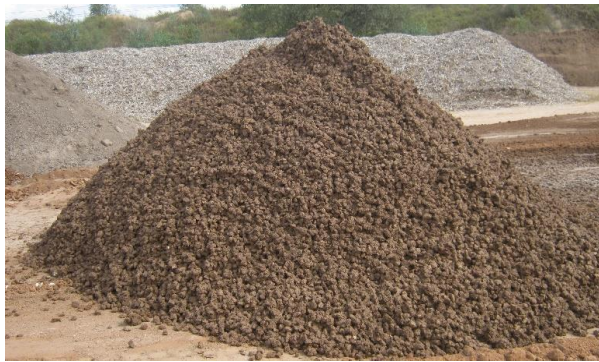
Clay loam soil is mixed with the crushed stone. The added Gelscape® Tackifier helps it “stick” and prevents settling during construction. Photo courtesy J-V Environmental Services
