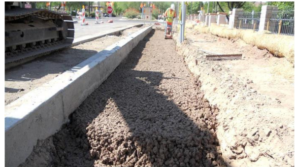
Compaction of CU-Structural Soil® during installation. For proper installation, CU-Structural Soil® must be compacted every 6 inches. Photo courtesy AZ Best, LLC
