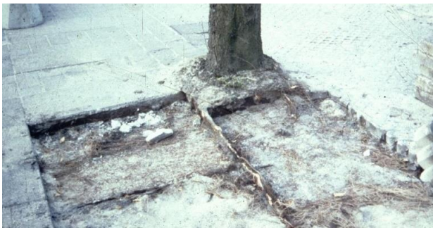
With paving removed, it is easy to see how this tree's roots took advantage of the weak points in the pavement. While the tree survived, the expanding roots caused the pavement to fail.
