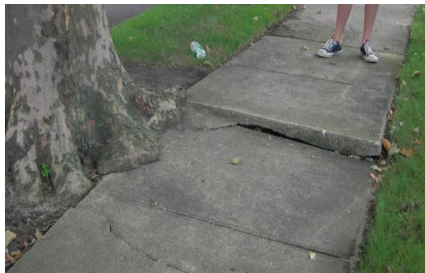
The roots of this tree have grown through the compacted soil beneath the sidewalk, into the large volume of soil beyond. Expanding tree roots have caused the sidewalk to heave.
