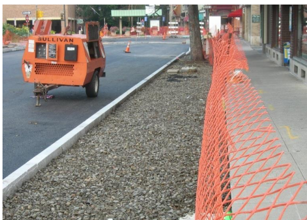
Installation of the new sidewalk on a base of CU-Soil®. This picture also shows an existing mature tree
