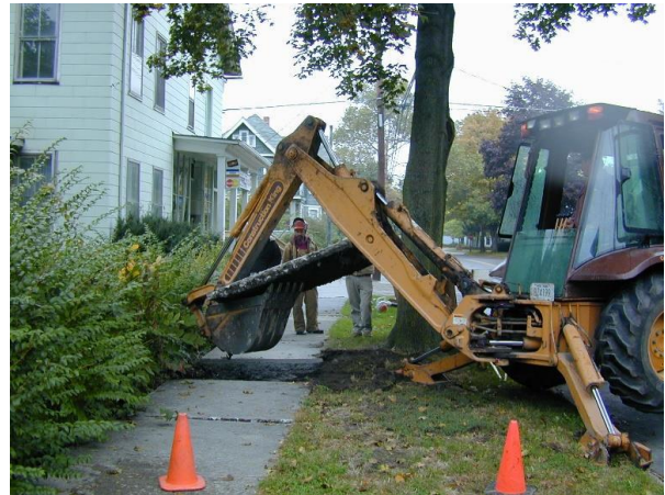
Removing this sidewalk section, and replacing it with one that has a CU- Soil® base, will allow tree roots to grow out from the tree lawn. Ithaca, NY
