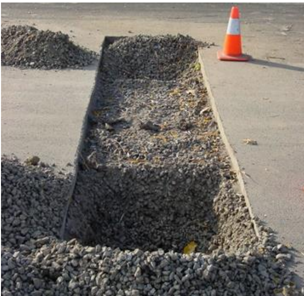
The saw-cut planting bed with holes dug in the CU-Soil® for tree planting.
