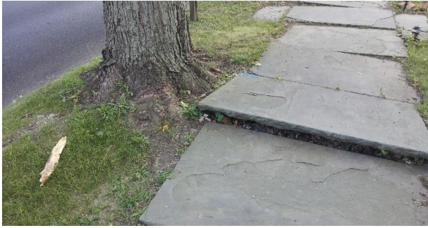
Tree roots heaving pavement
