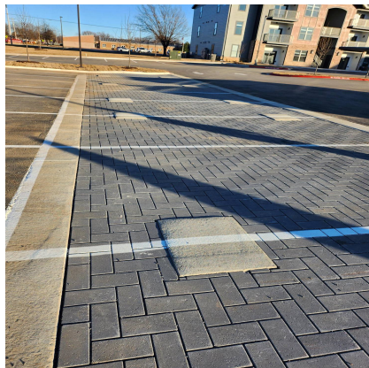
Photograph WQ-6 – Example of Permeable Pavers.
