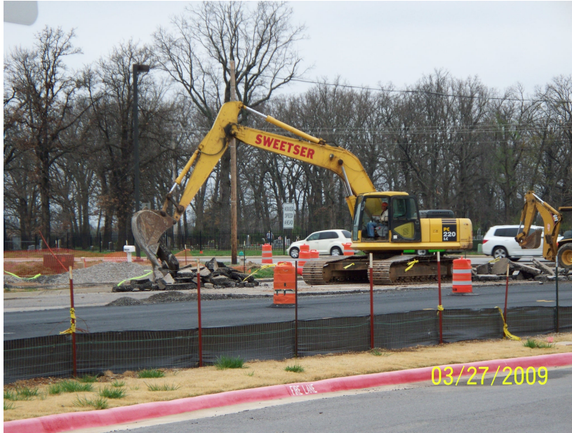
Photograph CS-4 – Example of Silt Fencing
