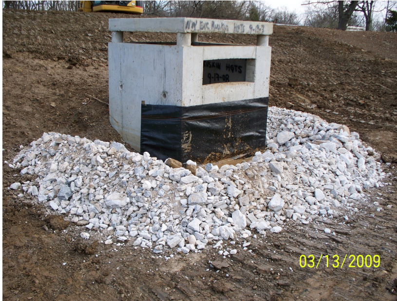
Photograph CS-5 – Example of Inlet Protection
