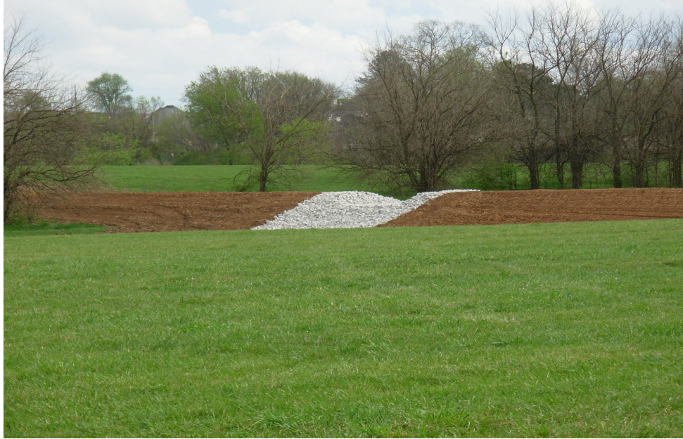
Photograph CS-6 – Example of Sediment Basin with Stone Outlet
