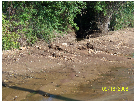
Photograph CS-1 – Example of Erosion during Construction
